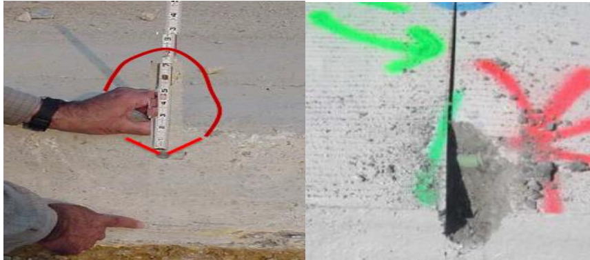
Figure 4: Bars placed at incorrect depths resulted in spalling (Khazanovich 2011: 45-46)
